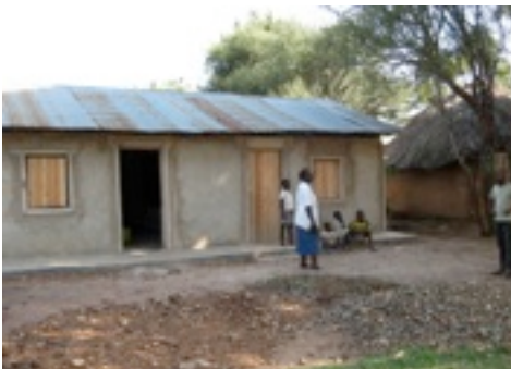
This building used to look a little worse than the typical school above. Here it is on the day we finished with the renovation.
