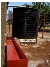
A rain-water system installed by Emerge at Pandpieri primary.
